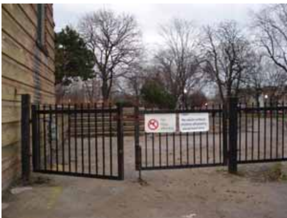
Figure 3 Broken Latch – rusted fencing; there are spaces between fence's bars wide enough for a child's head or part of body to become stuck
